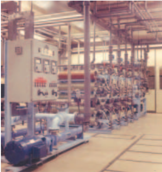
FIG. 21. High-pressure multi-stage pumping station of the 60 m 3 /h hollow fibre reverse osmosis plant.
