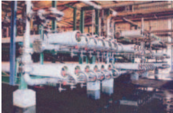
FIG. 22. Fixed membrane reverse osmosis system with a throughput of 240 m 3 /h.
