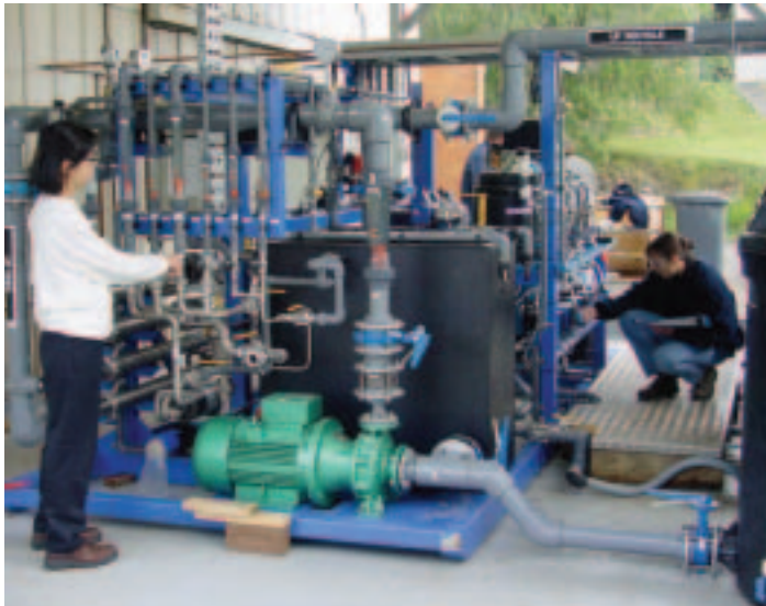
FIG. 19. Two views of a skid mounted pilot plant containing tubular ultrafiltration and spirally wound reverse osmosis systems (courtesy of ANSTO).
