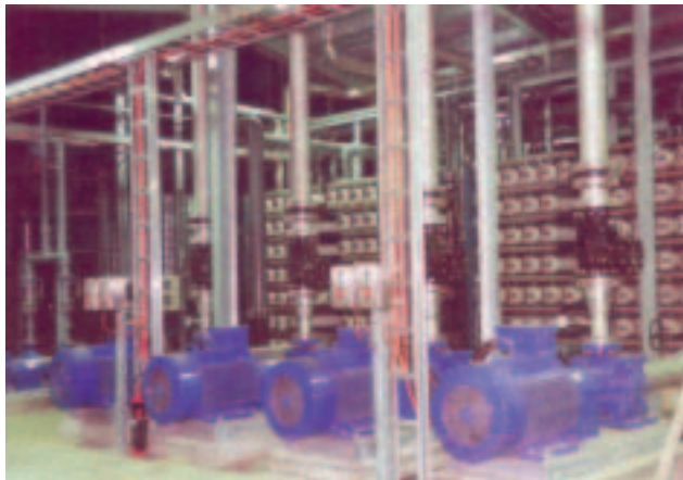
FIG. 23. Fixed membrane ultrafiltration/reverse osmosis system with a throughput of 670 m 3 /h.
